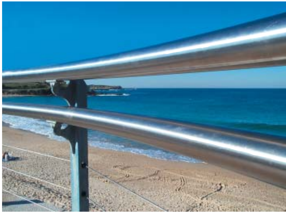
Figure 1: Successful use of stainless steel, after more than 10 years service, in a coastal environment.
