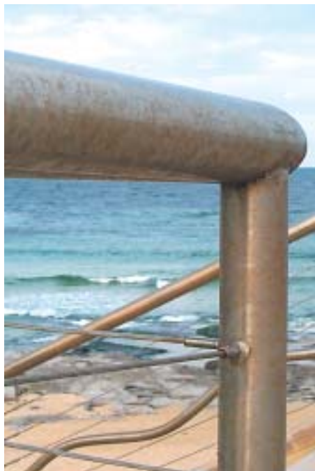
Figure 2: Tea staining of stainless steel in a coastal environment shortly after installation.
